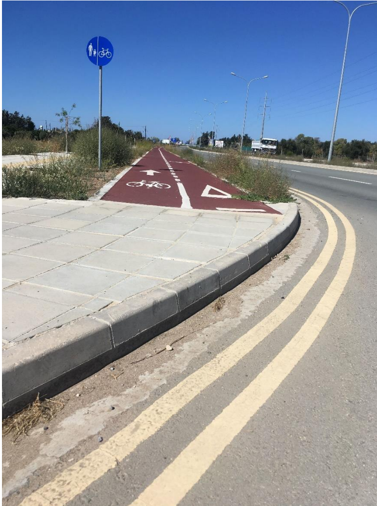
High kerb at the edge of a segregated cycle path in Pafos
